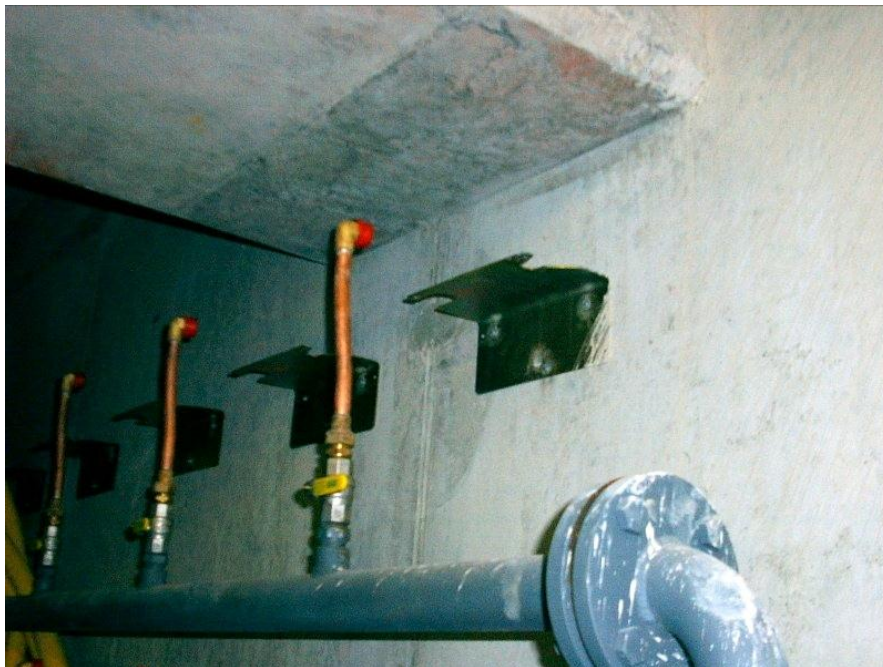
Fig 9 Typical gas manifold and bracket arrangement for the installer who runs pipe to bracket slot.
